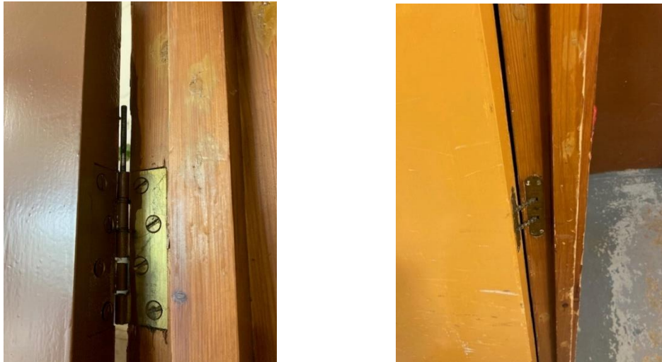
Figure 2 Defective fire door hinge and Perco closers.
