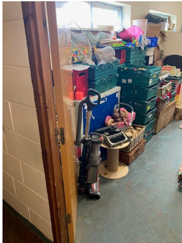
Figure 1 Fire door to storeroom held open onto escape corridor.
