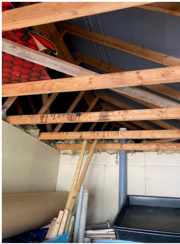
Figure 3 Fully exposed roof materials above combustible items in garages.
